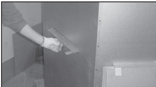
Figure 3.7 Bend Refractory Brackets Back Down
