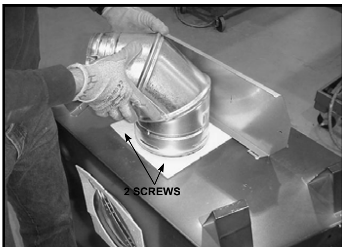
Figure 6.11 To attach the first section of vent pipe, make sure to use the fiberglass gasket to seal between the first vent component and the outer fireplace wrap. Use 2 self tapping screws to secure the gasket to the outer wrap.
